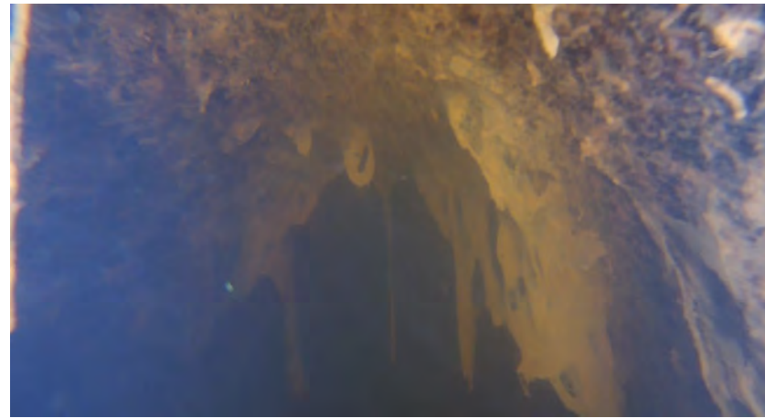
Photograph 2: Marine Growth Observed at the Obvert (top) of the Intake Pipe
